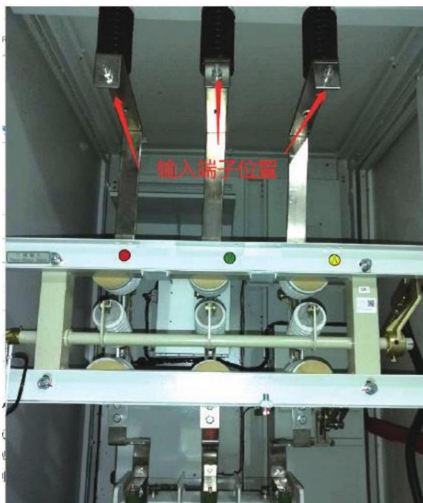
Figure 6.8 Three-phase main cable connection terminals
